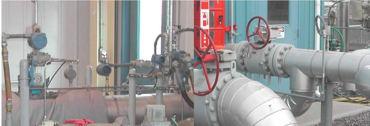
Turbine Meter and Instrumentation
