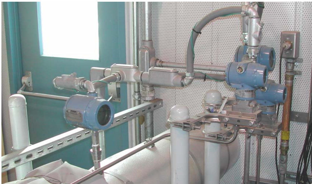
"Redundant" Temperature and Pressure Transmitters
